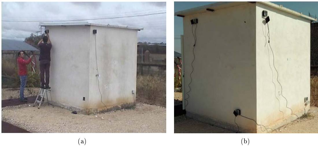
Figure 3.6: Installation of the sensor nodes on the different outdoor façades of the building during October 2014.
