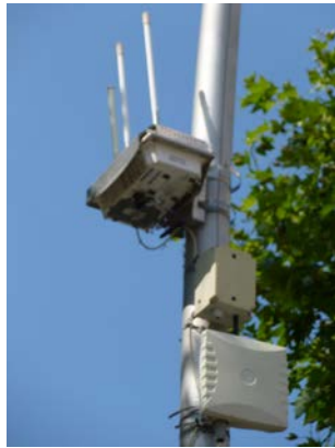
(a) The sink node, as mounted during the experiments.
